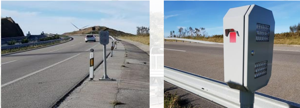
Illustration 45. Beacon installed on the A-8 motorway. Source: DGT
