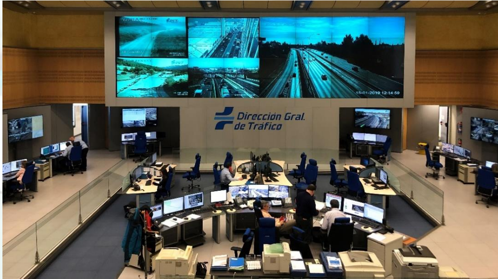
Illustration 76. Traffic Management Centre in Madrid. Source: DGT
